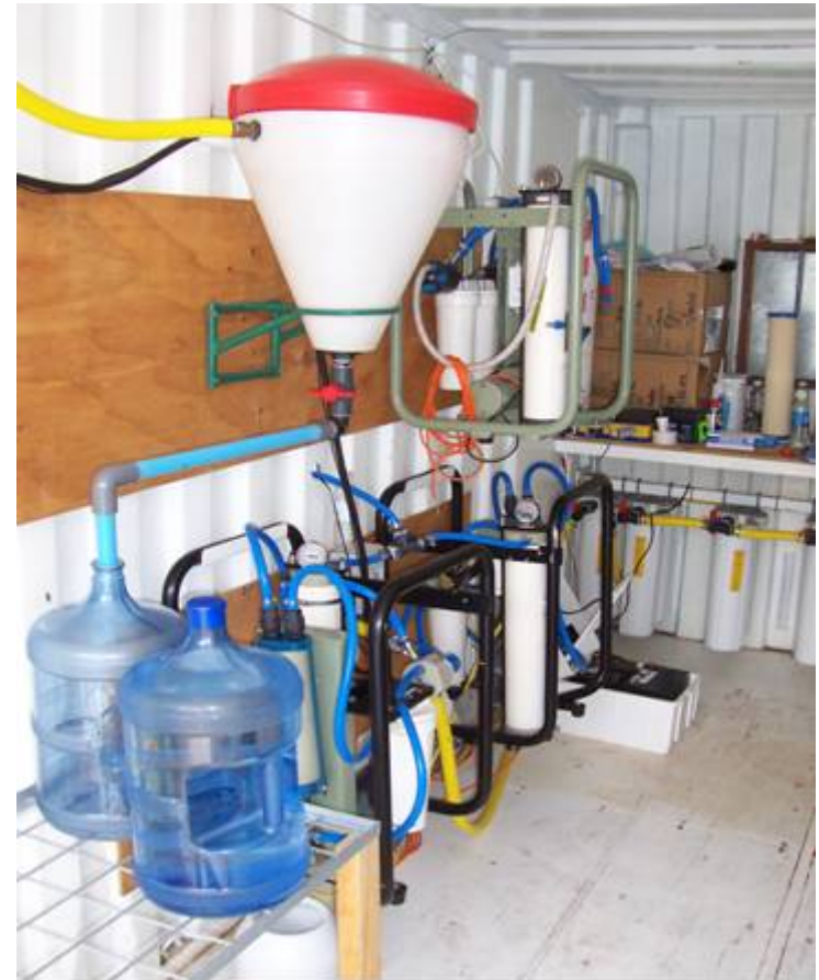
Purification equipment inside the container
