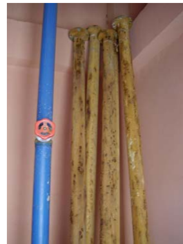
Used corroded metal pipes
